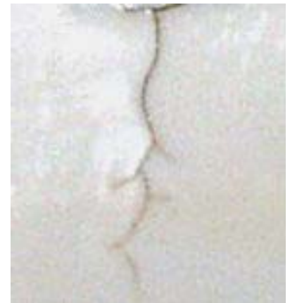
Swelling is clearly apparent in this picture of 'structural' damage
