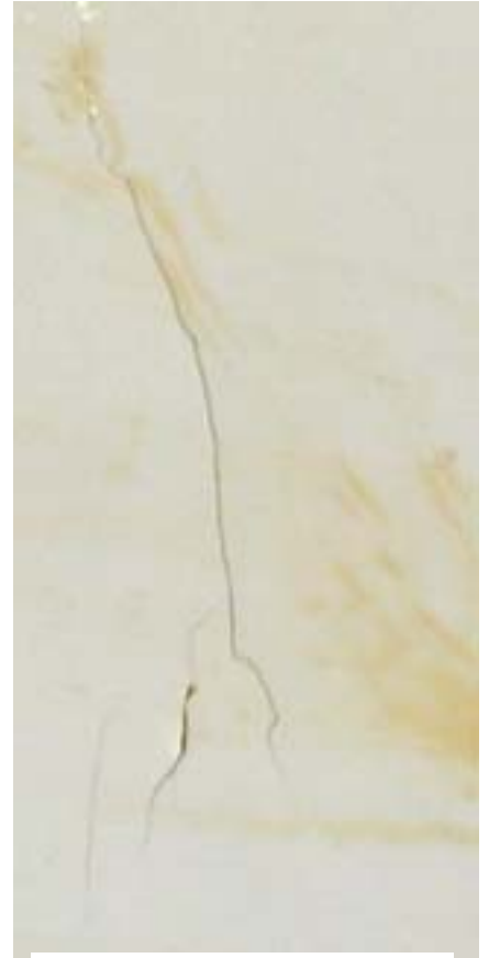
Another view of a superficial crack.
